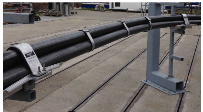
A photo of the short circuit test rig for Centaur Trefoil including Flexi-Straps (see page 28). Testing was carried out at ZKU Laboratories in Prague, CZ.
