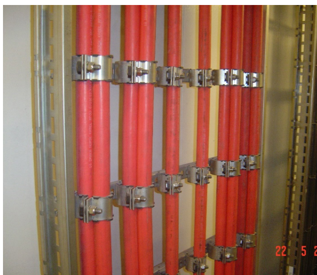
THE AXIAL LOAD RATING OF A CLEAT IS USED TO SPECIFY THE SPACING OF CLEATS TO HOLD THE WEIGHT OF THE CABLE IN VERTICAL INSTALLS
