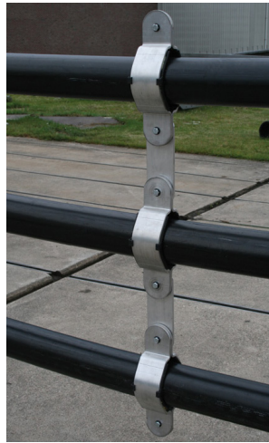
TYPICAL INSTALLATION, PHOTO TAKEN AT A SHORT CIRCUIT TESTING EVENT AT KEMA LAB, ARNHEM NL
