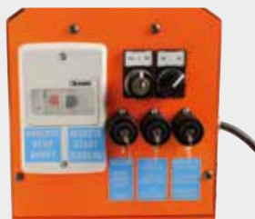
Front panel electric control unit
